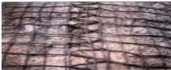
Figure 4: Boulder net laid on Konkan railway line [23]
